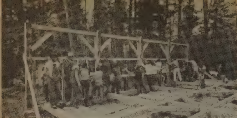
Temporary braces are applied to the bent to stabilize it. The opposite wall bent, lying in the foreground, is next. The remainder of the timbers are carefully stacked according to their placement in the frame.
